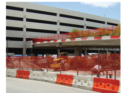
Garage & Parking Lots
